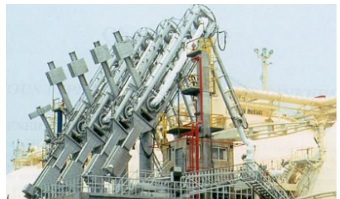
Figure 7. Unloading arms at an import (receiving) terminal (Source: BV 2009)
