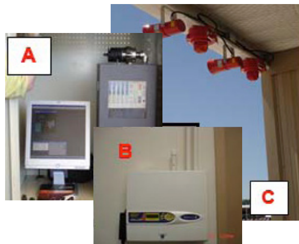
Figure 2. Detection and warning devices for LNG terminals: A) flame detection monitoring in a control room, B) aspirating smoke detector, and C) audible alarms
